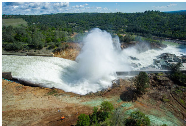
Flood waters pour out of Oroville Reservoir, scouring the spillway and hillside, and causing major evacuations in California, 2017. Credit: DWR.
