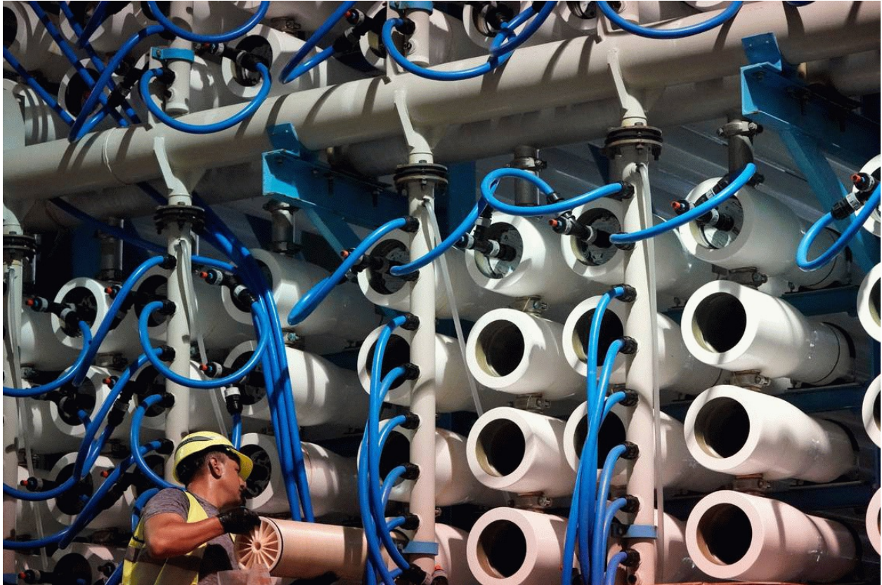
A man performs maintenance work in the reverse osmosis building at the Carlsbad Desalination plant in May in Carlsbad. The facility is the Western hemisphere's largest desalination plant, which removes salt and impurities from ocean water. Gregory Bull AP
