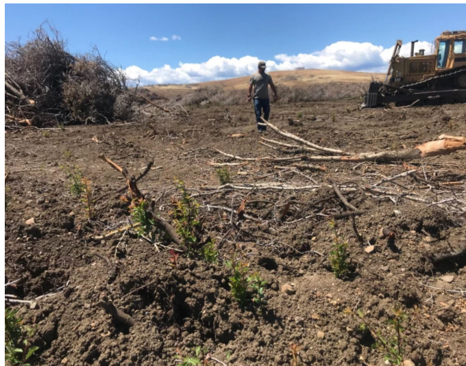
"I had no choice," said Zachary Dennis about bulldozing 377 acres of almond trees. "Our water allocation dropped to zero, and the price of water from contractors jumped to $600 an acre-foot — about six times what it costs in normal years." (Louis Sahagún / Los Angeles Times)
