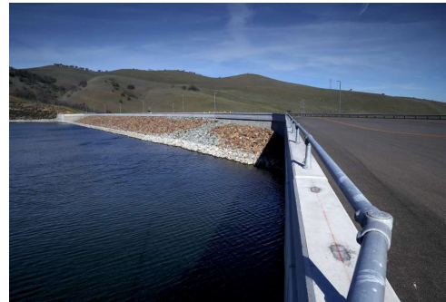
The dam at Los Vaqueros Reservoir in Brentwood, Calif., on Friday Feb. 2, 2018. More than a dozen local water agencies are trying to tap a windfall of state funds to expand Los Vaqueros Reservoir into a regional giant that serves San Francisco and Silicon Valley.
