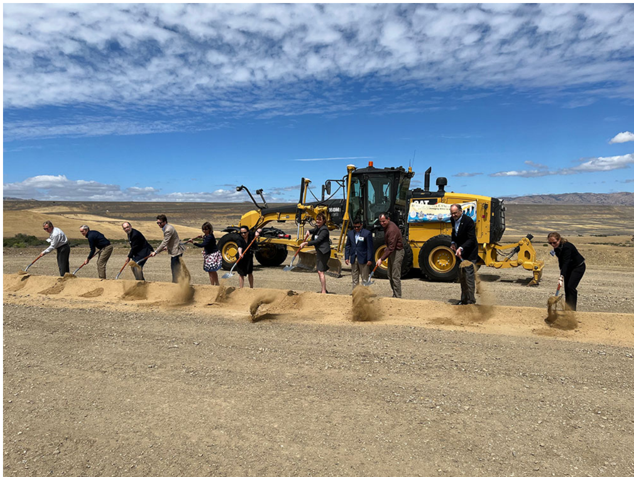
Dirt is turned on the B.F. Sisk Dam Safety Modification Project today. Event held to kick-off Reclamation's 120th Anniversary today.
