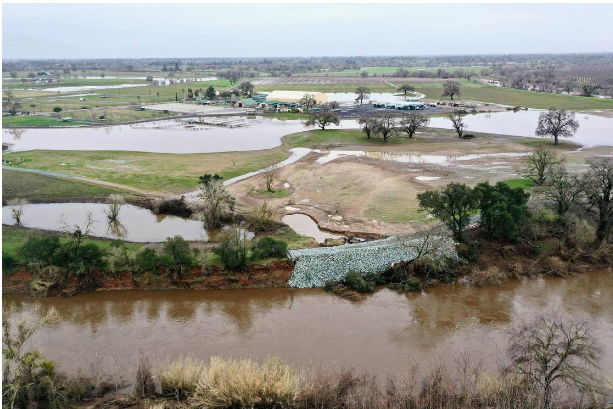
A repaired Cosumnes River section of levee, where a break earlier this month caused flooding in Wilton, awaits the test of another storm on Monday. Hector Amezcua hamezcua@sacbee.com
