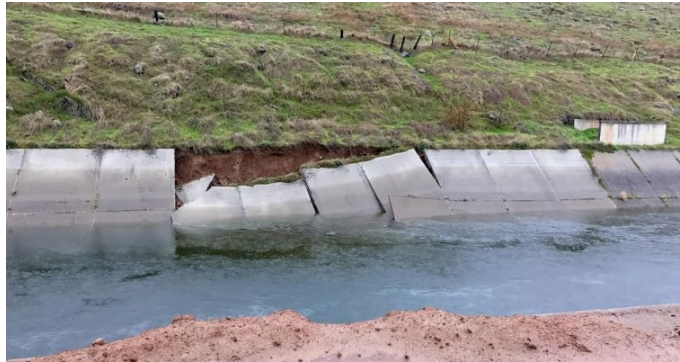
The Bureau of Reclamation is funding repairs on the Friant-Kern Canal. (friantwater.org)
