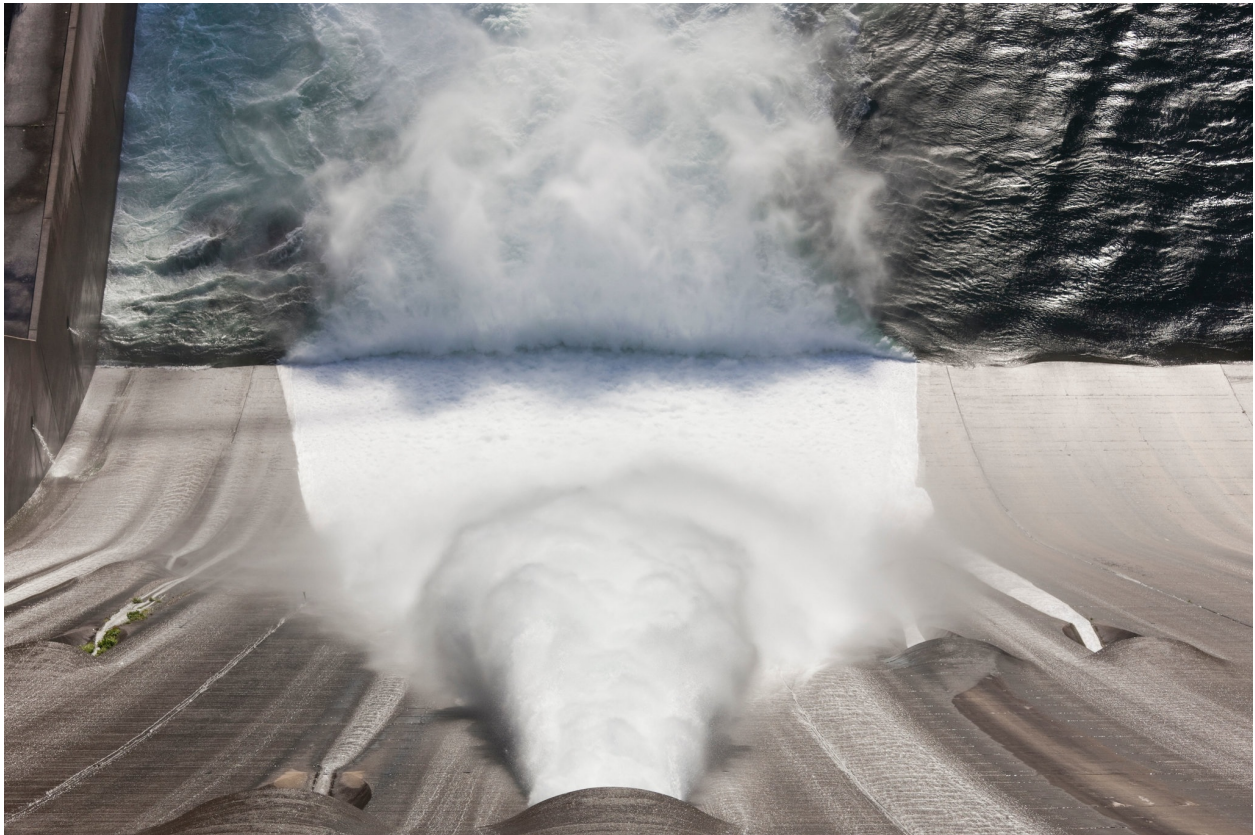
The spillway of the Shasta Dam in Northern California. Walter Bibikow/Denita Delimont, via Alamy
