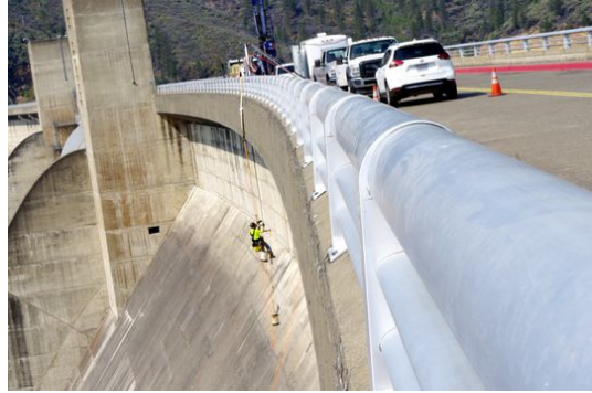
Workers did testing on Shasta Dam in 2018 to determine whether it could withstand having an additional 18 1/2 feet of concrete placed on the crest of the dam. (Photo: Damon Arthur/Record Searchlight)
