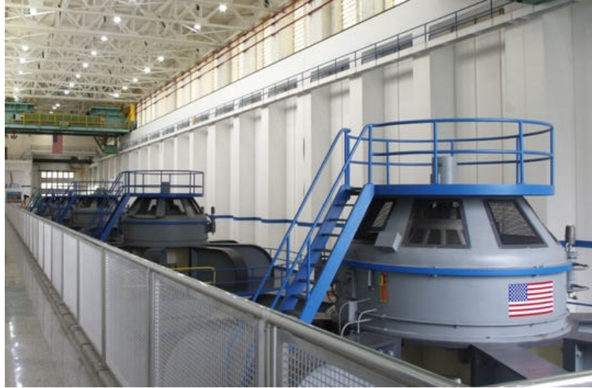
File - In March 2019, four of the five turbines below Shasta Dam were turning, creating electricity. (Photo: Damon Arthur/Record Searchlight)
