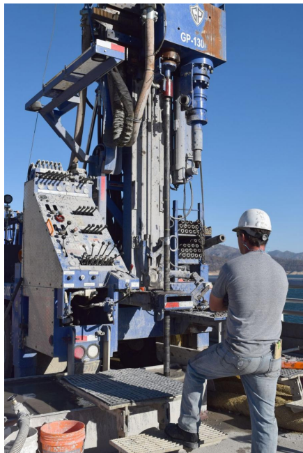
Samuel Thomas, drill operator from Reclamation's Boise office, is drilling core samples.
