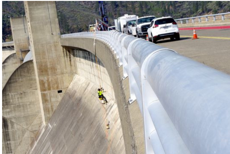
In September 2018, Nathan Morgan hangs over the side of Shasta Dam. Morgan and others were drilling holes in the dam to test the strength of the concrete in preparation for raising the height of the dam. (Photo: Damon Arthur/Record Searchlight)
