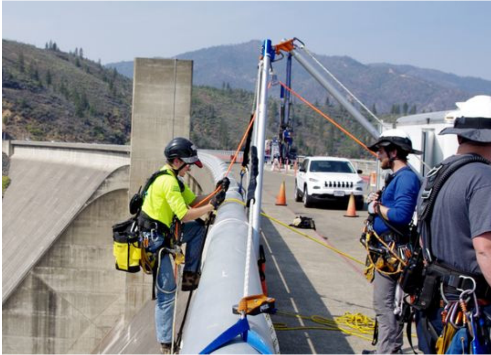
Nathan Morgan climbs back on top of Shasta Dam in September after doing work to prepare for drilling holes in the dam. The holes were being drilled to test the strength of the concrete in preparation for raising the height of the dam. (Photo: Damon Arthur/Record Searchlight)
