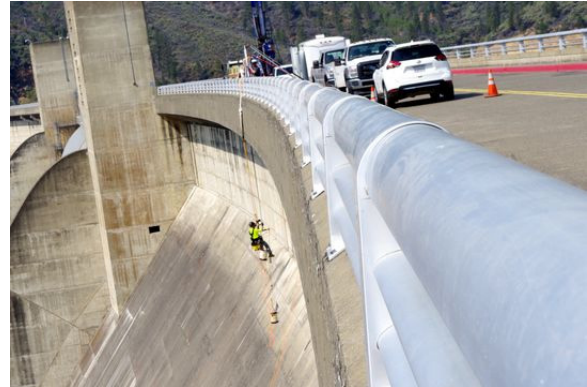
Nathan Morgan hangs over the side of Shasta Dam on Thursday. Morgan and others were drilling holes in the dam to test the strength of the concrete in preparation for raising the height of the dam. (Photo: Damon Arthur/Record Searchlight)
