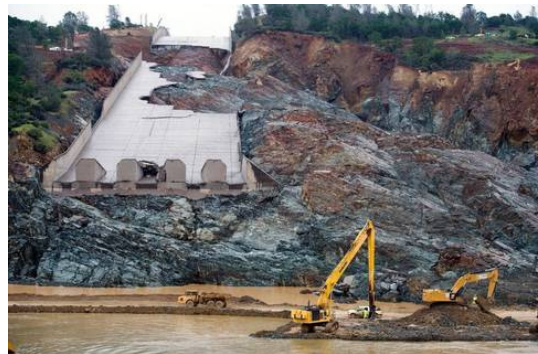
The wreckage of the main spillway at Oroville Dam in February 2017 left tons of concrete and other debris piled up in the Feather River below. Randy Pench Sacramento Bee file
