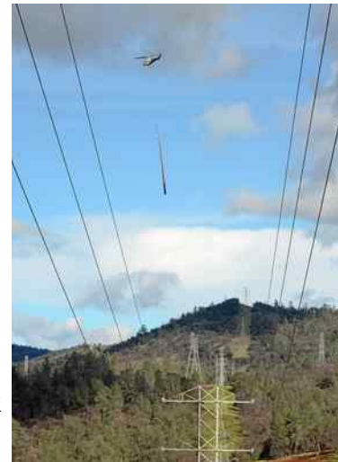
Helicopters haul power poles by air as PG&E crews remove towers along the Diversion Pool to reroute transmission lines on Feb. 22, 2017 at the Oroville Dam. Dan Reidel — Enterprise-Record file photo
