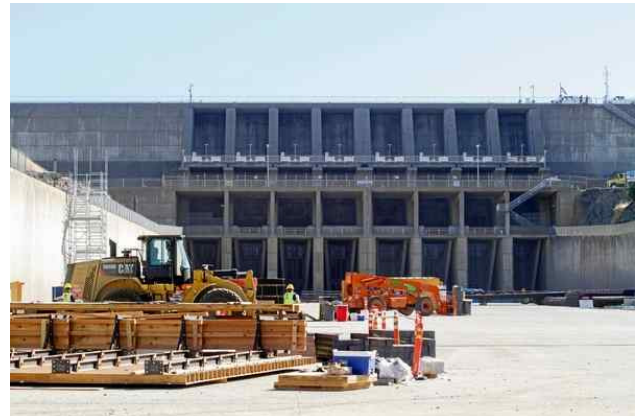
The spillway gates are seen from the other side of the lake, from the spillway itself, as construction continues on July 7, 2017. Emily Bertolino — Enterprise-Record file
