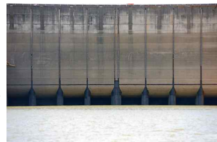
The Oroville Dam spillway gates, near the waterline in this photo taken from the lake on April 1, 2017, were in danger of being inoperable during the spillway crisis. Dan Reidel — Enterprise-Record File
